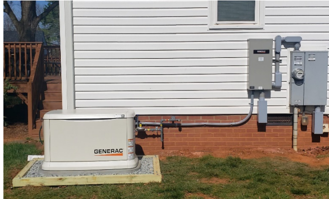
Whole House Generator
