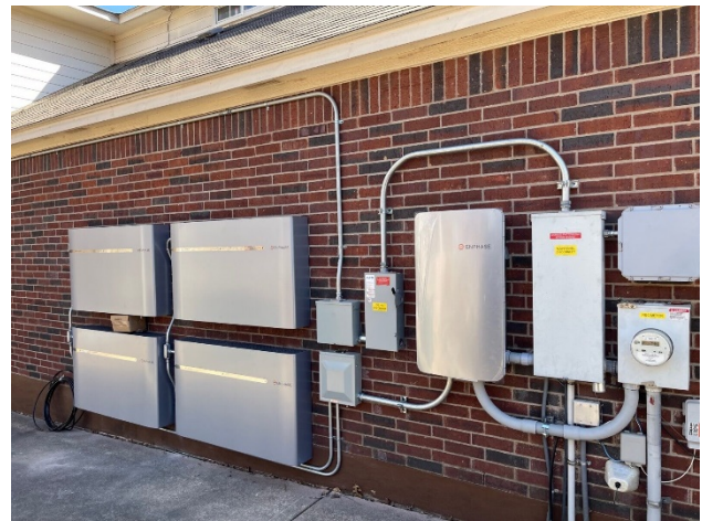
Whole House Battery Storage System
